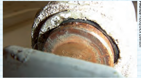
A closer look shows this brake unit was only a few applications away from failure.
