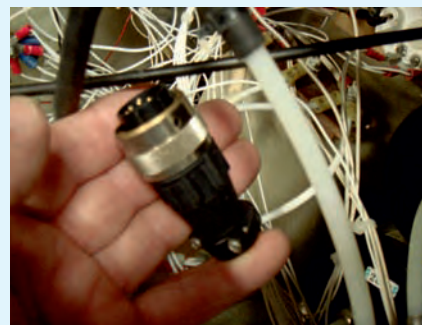
Actual socket that came apart leaving LAA test pilot without an engine. We used to call this 'spaghetti' wiring when we were younger.
