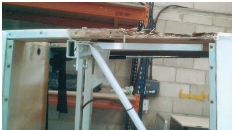
Fig. 1. (Opposite) Shows the damage found to the port lower longeron when the lower fuselage inspection panel was removed. This picture was taken after the wings and tailplane had been removed and the aircraft laid on trestles on its side.
