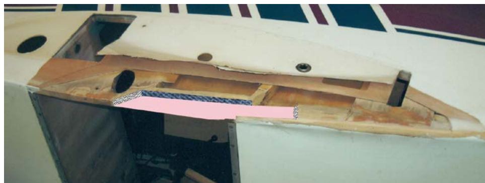
Fig. 2. This picture shows well the extent of the damage; in this picture the repair team has removed all the damaged wood revealing just how much of the structure was compromised.
