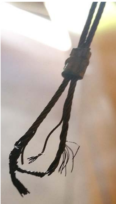
Fig. 2. This close up shows the extent of the damage found by the engineer when the cable was removed from the 'U' clamp. The point of bending is clear.
