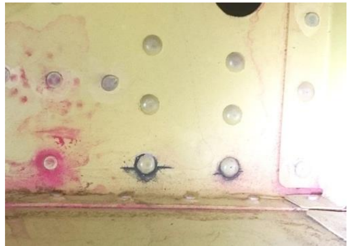
Fig. 1. Cracking of wing aft. spar web at the inboard aileron hinge. This picture, taken from the Service Bulletin, shows a view taken from inside the wing (looking aft.). (Courtesy of Vans Aircraft).
