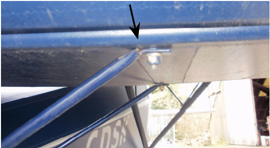
Figure 3: View from rear of horizontal stabiliser (elevator raised) showing crack at flattened end of strut.
