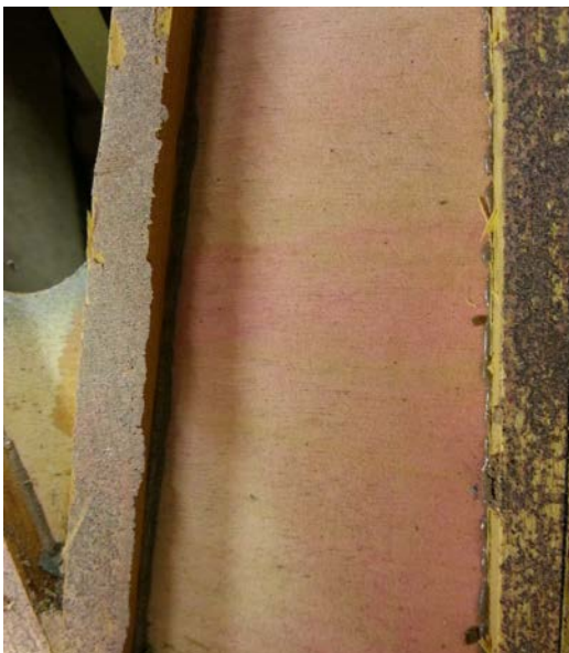
Fig. 2 A closer look at the failed glue joint reveals that the actual failure appears to have occurred along the wood-activator joint (not shown); the resinous joint appears still to be functional. (Courtesy of BGA).
