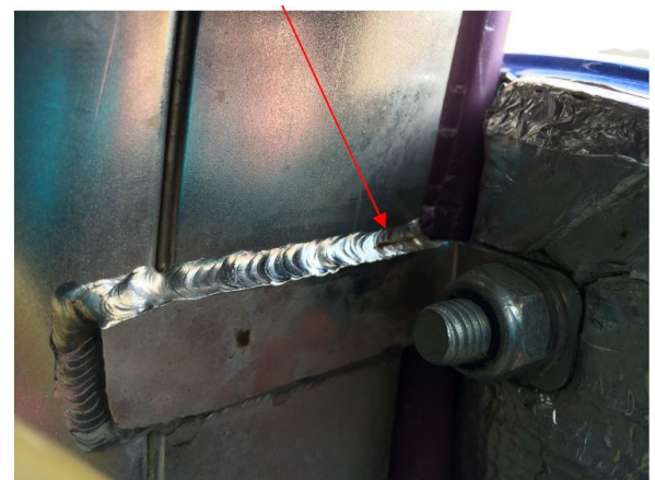
Fig 3. The recent Rotorsport SIL gives examples of cracks that engineers have spotted in welded joints in the structure; the crack shown was found in the right hand upper body bracket. Cracks like this, when spotted early, can be easily repaired, but if left can result in expensive structural repairs.
