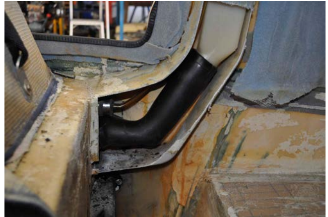
Fig 1. Picture shows the fuel filler pipe in situ , note that in this example the pipe was completely hidden inside the fibreglass enclosure.
