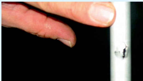
Frame tube crack on a Rans S6 - was it caused by ice forming within the tube, or something else?
